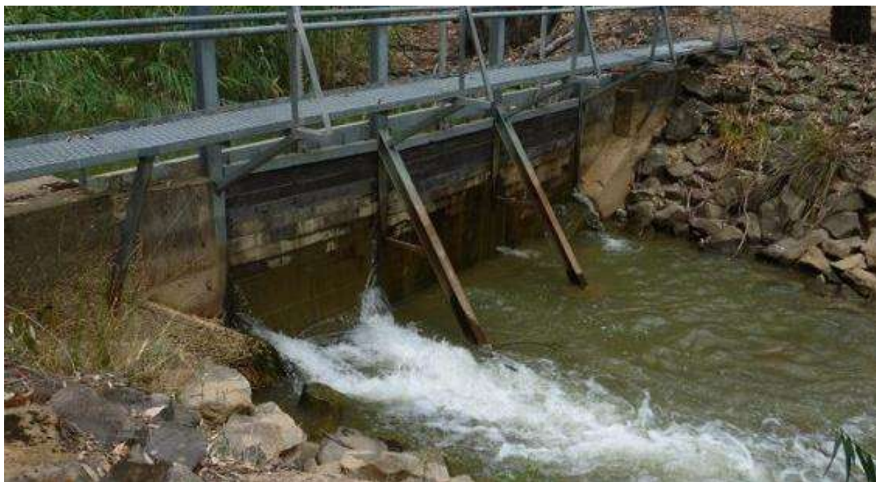
Photo 2-5 Existing Nestrons regulator, downstream side, showing leakage through the fully closed gates
