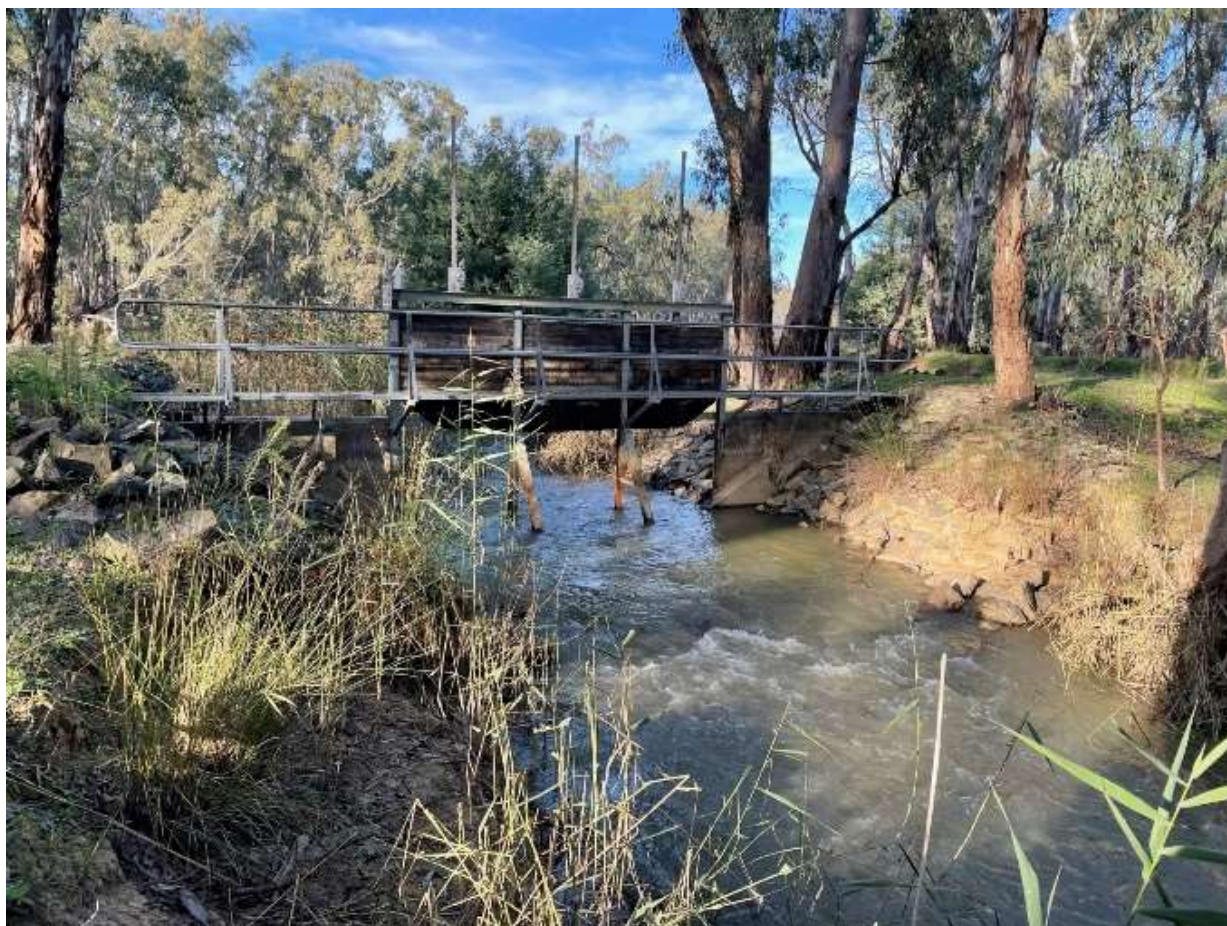
Photo 2-7 Existing Nestrons regulator, downstream side, shortly after opening of the gates
