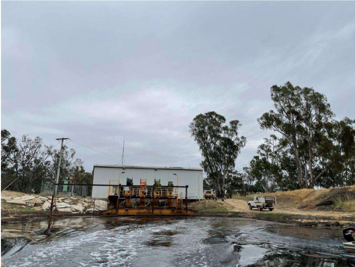
Photo 2-9 Pumps to extract water from the Murray River at Moira Creek to supply the MPID
