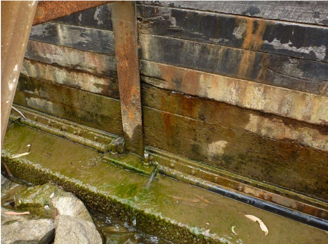
Photo 2-4 Water leaking through the gates on the existing Pinchgut regulator
