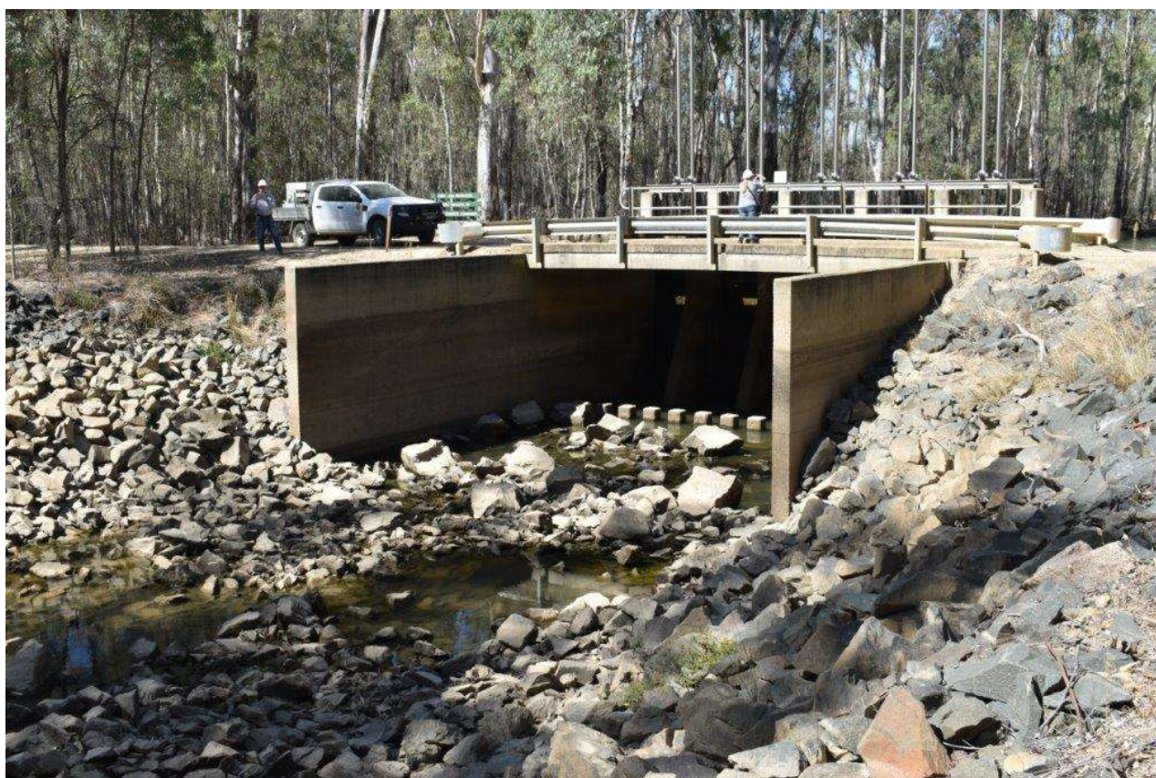
Photo 6-2 Mary Ada regulator, downstream end
