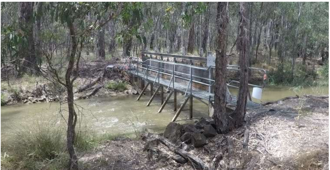
Photo 2-1 Existing Pinchgut regulator passing flows
