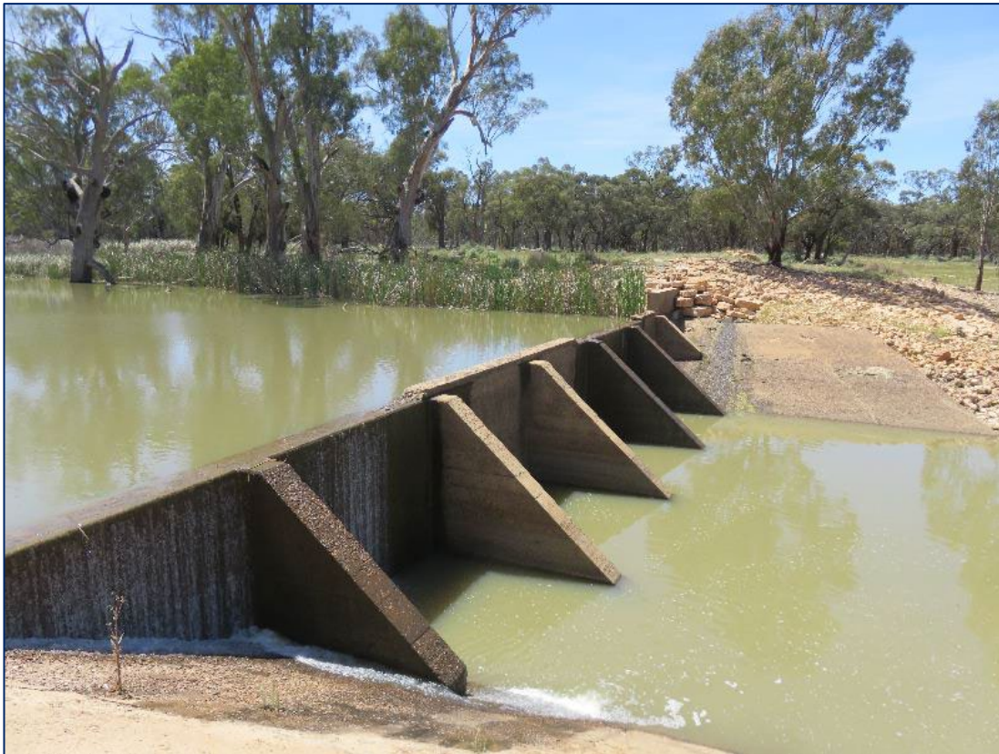
Figure 2-1 Existing Carrs weir No.1 structure (with piping leaks on left downstream abutment)
