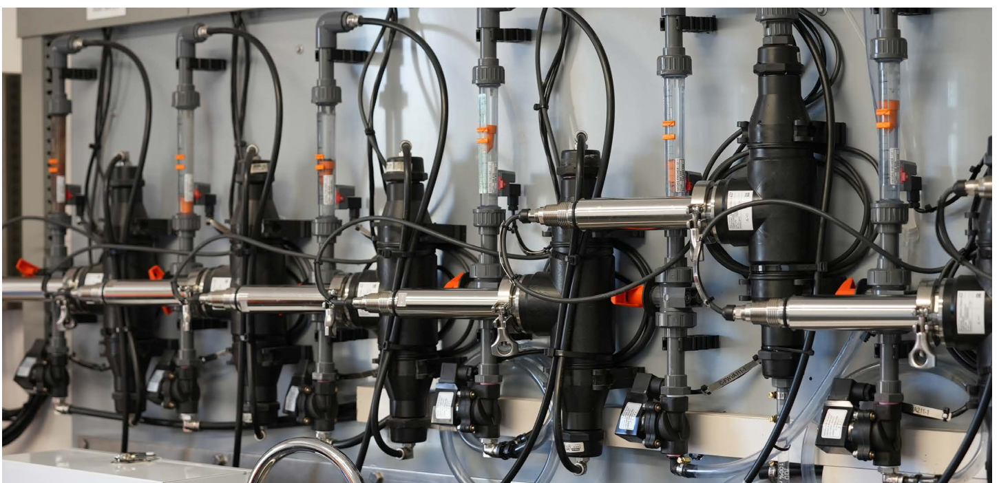
Image: Inside a water treatment plant in regional NSW. Photo: Vince Bucello.
