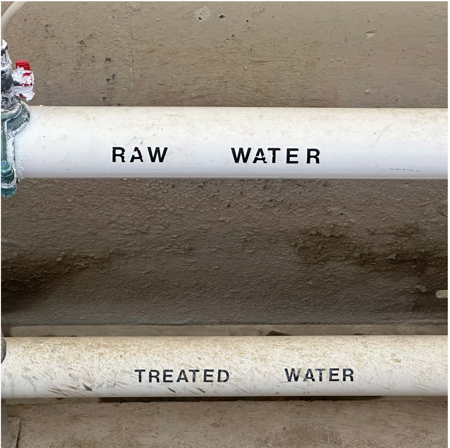
Image: As part of the water treatment process, raw and treated water must be kept separate.
