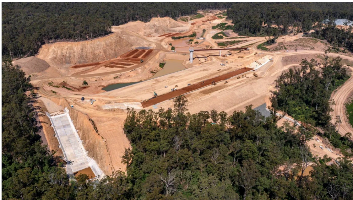
Aerial view of Eurobodalla Southern Storage Dam taken in March 2025. Credit: Eurobodalla Council
