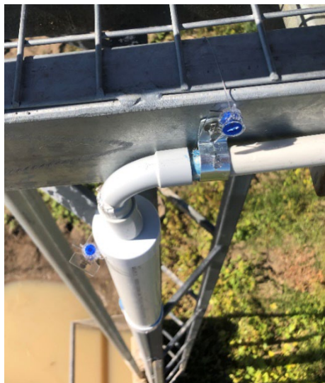
Figure 5. Image shows a tamper evident seal fixed to a pressure sensor on a catwalk
