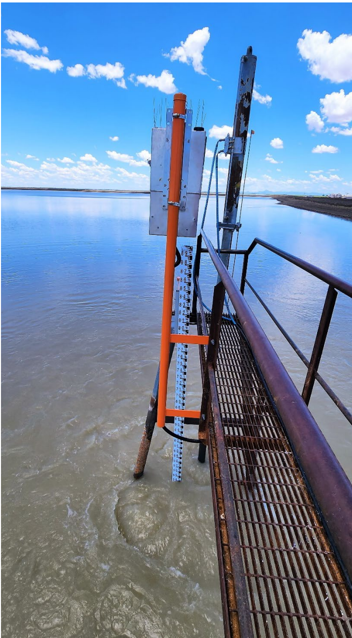
Figure 1. Depth gauge board installed on an elevated walkway
