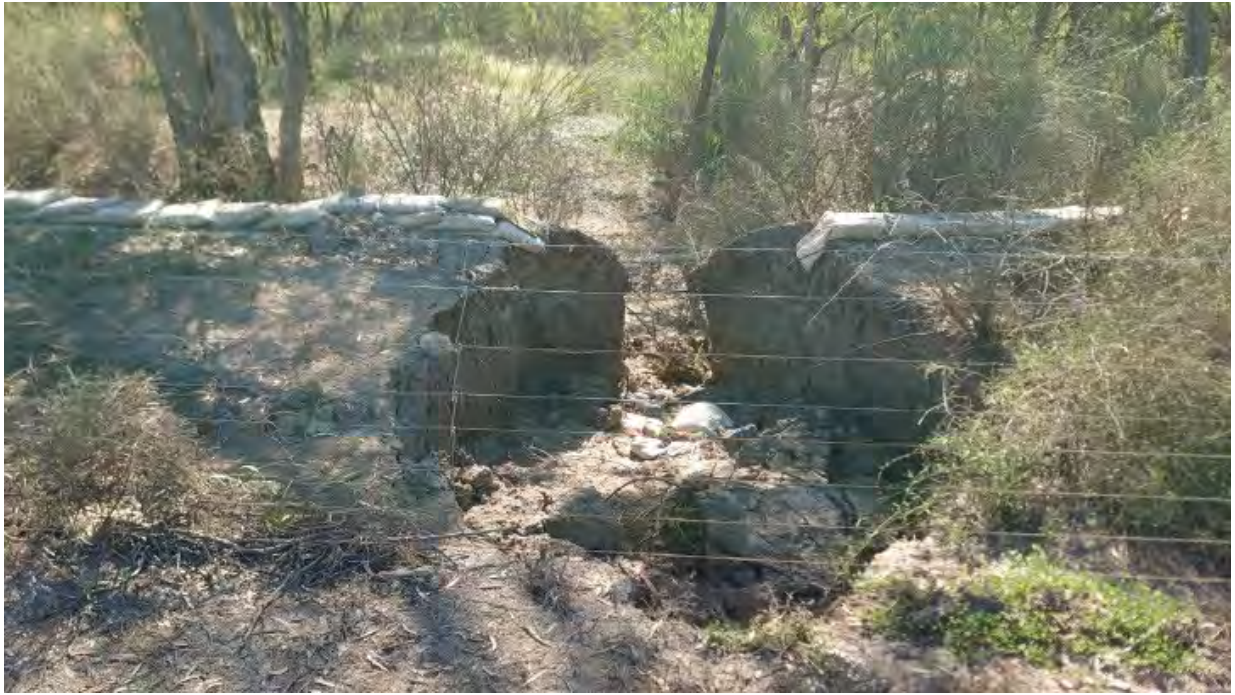
Image 9c :Breach in the [REDACTED] post flooding 2022/2023.
