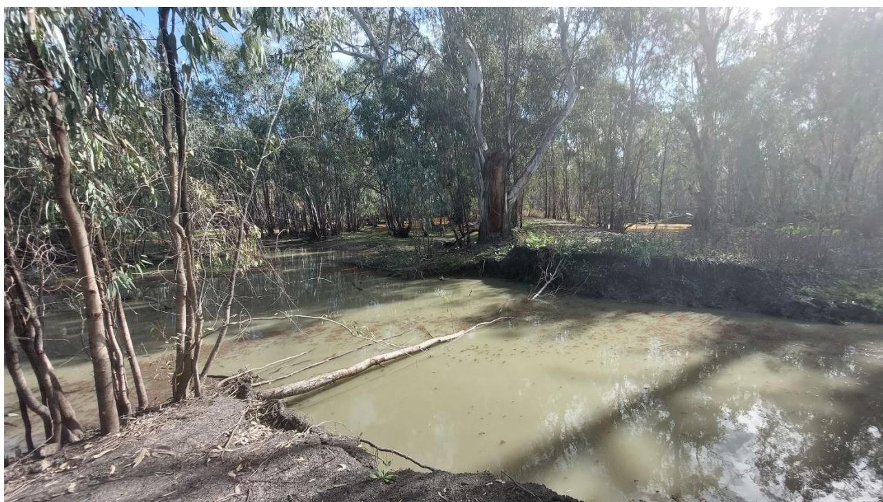
Figure 6-4 Recent (2023) breach in the levee bank on Steves Bank Trail (Buster's bank) on Narkungerie Creek
