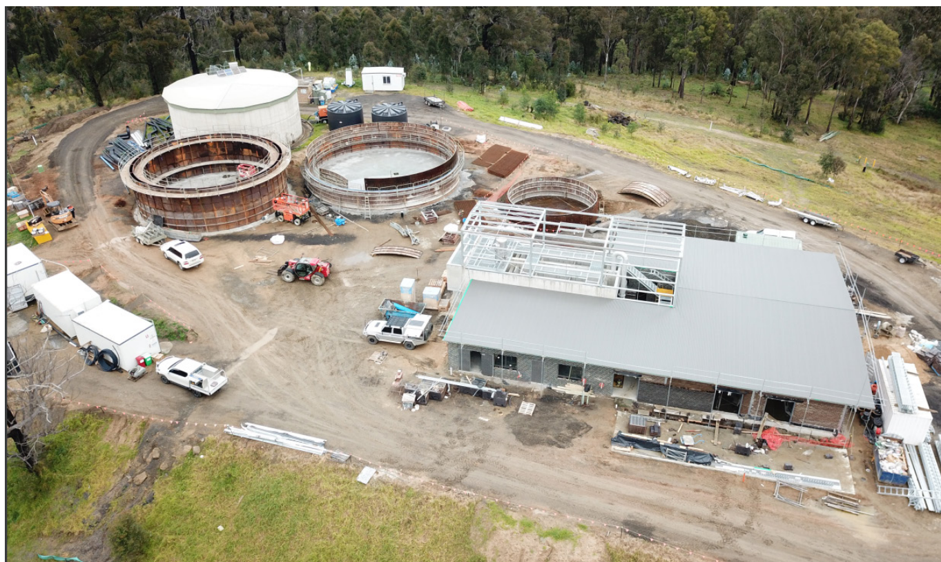
Brogo Bermagui Water Treatment Plant, NSW
