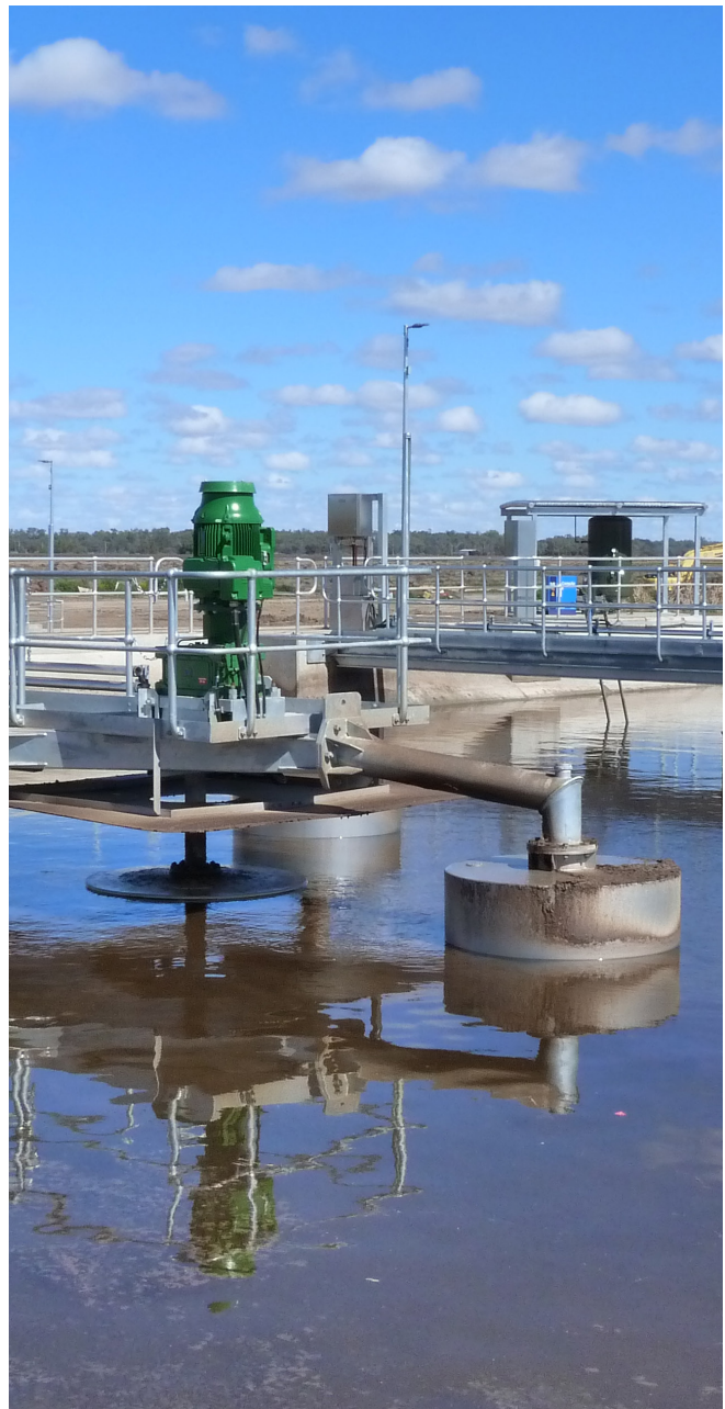
Hay Sewerage Treatment Plant, NSW
